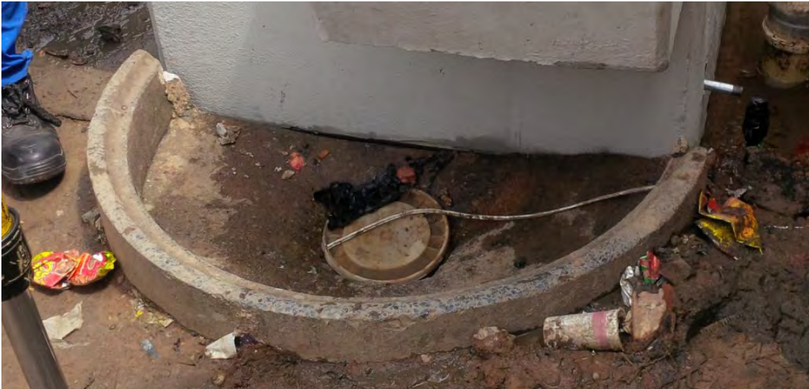
A typical existing waste water collection point (gully) connected to the sewer.
