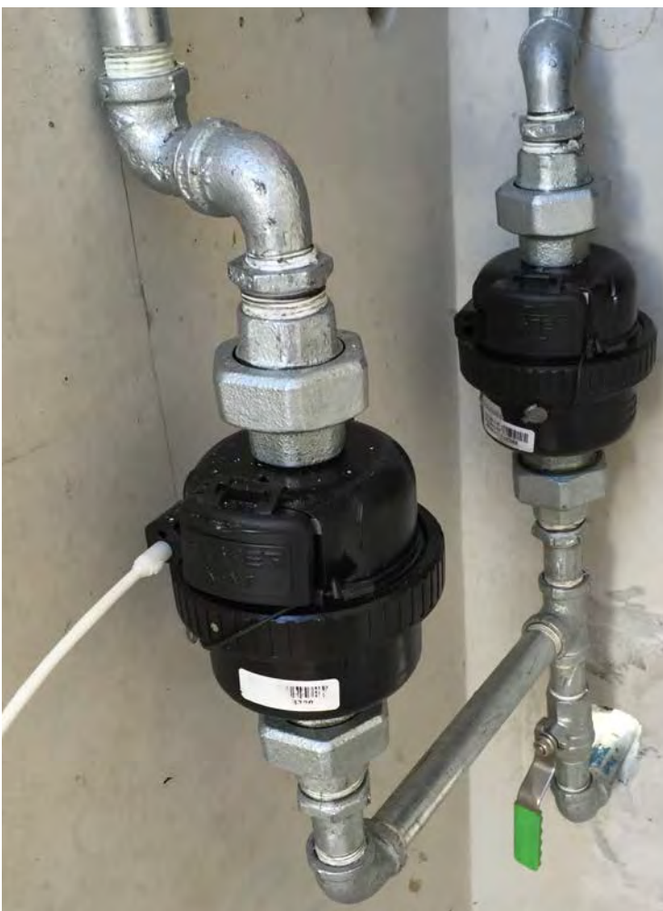
Water meters installed in March. One has a logger probe installed (white cable, left).
