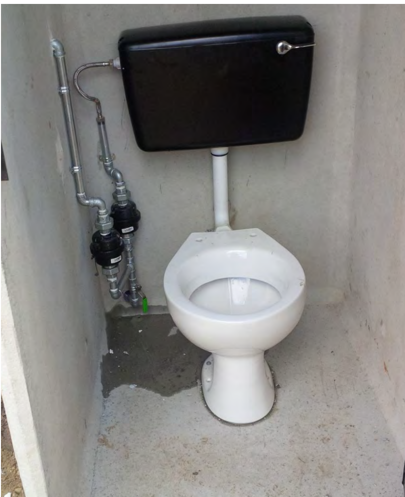
Water meters, pipework, pan and cistern used in March.
