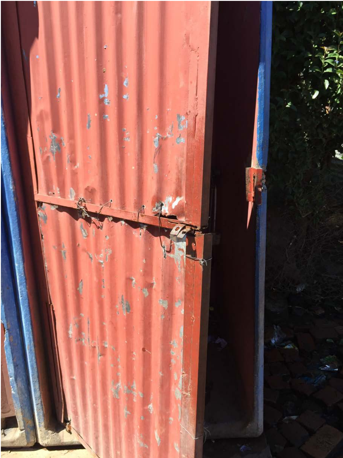
A failed door design that was trialed 2 years ago. Broken through the edge.
