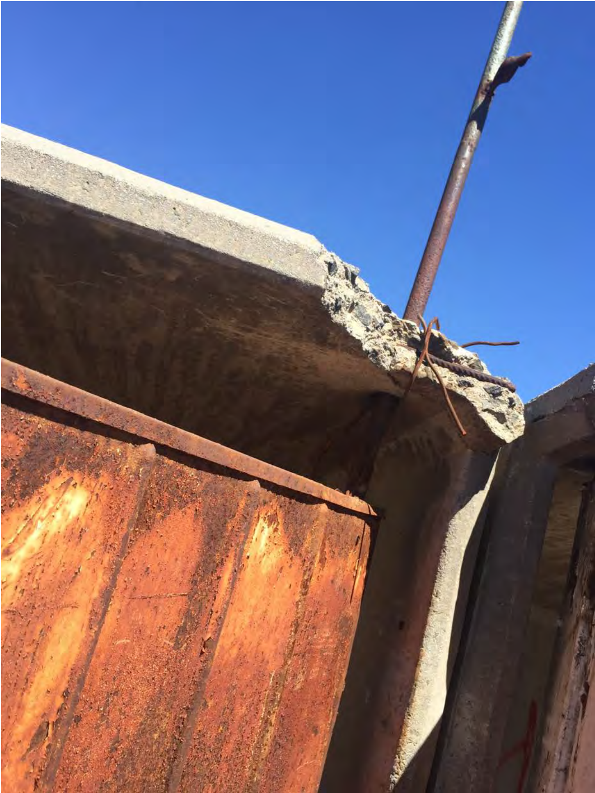
Typical damage to the top of unit near door hinge.
