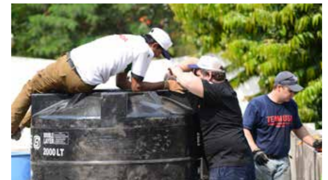
Members of Team India (Lalit Kasawate), Team Australia (Aaron Bridger), and Team USA (Adam Koenigs) work together on the school roof to install a new water tank that will supply the upgraded handwash area. Credit: Anill Patil
