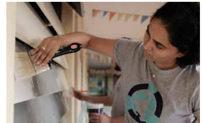
Swathi Saralaya of IAPMO India puts the finishing touches to new louvres added to help improve light, ventilation and privacy for the boys and girls toilets. Credit: Alan Gwee
